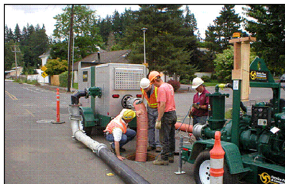
Upper Interceptor, Bypass Pump Test
