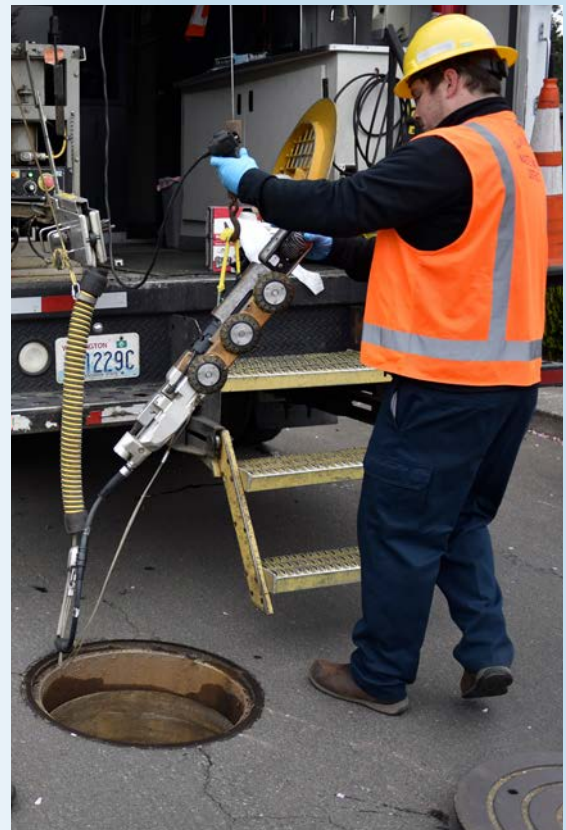
Staff place a CCTV camera into a manhole to inspect sewer conditions.
