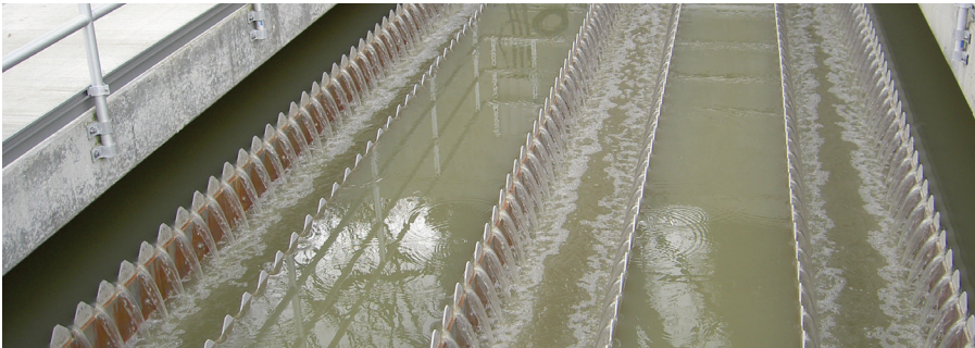
Wastewater flows through a primary clarifier at the Salmon Creek Treatment Plant
